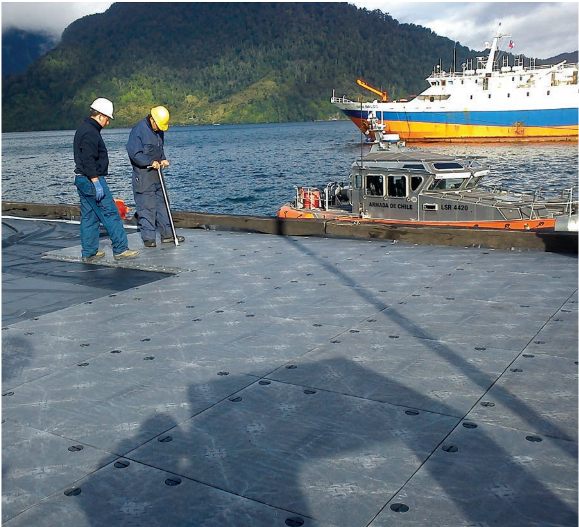
Be sure to lock each panel as it is set in place.
