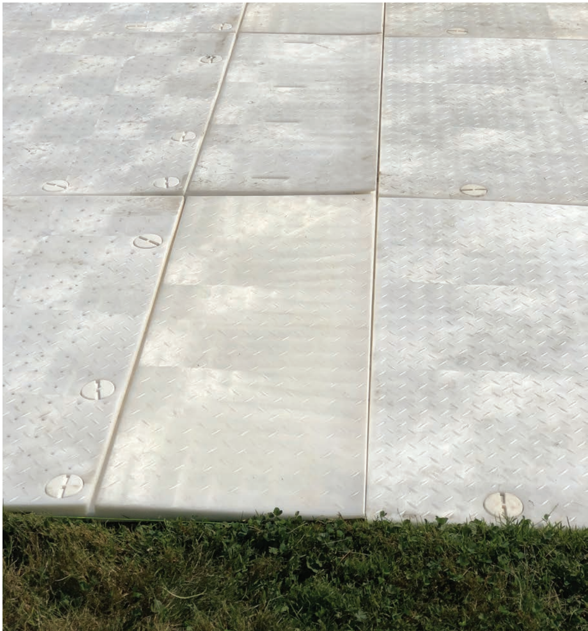
The leading edge of the HD/LD build joint is flush with the panels being adjoined.
